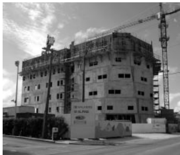
Construction on the 100,000 square-foot Walkers Building is well underway as the private sector continues to invest in the infrastructural development of Grand Cayman.
