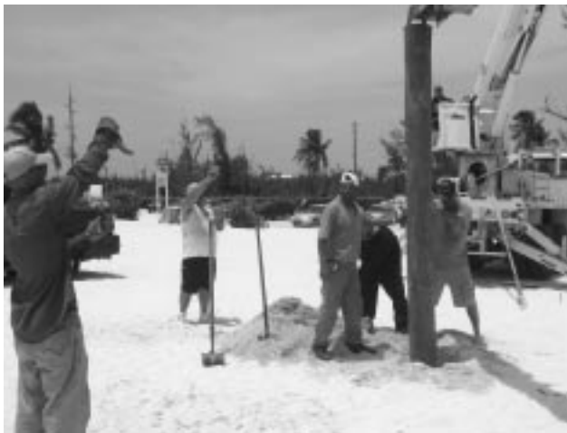
CUC and MasTec crews install poles for new cabanas at the popular Seven Mile Public Beach. The Company also began the refurbishing of the playground at the beach, which was damaged by Hurricane Ivan.
