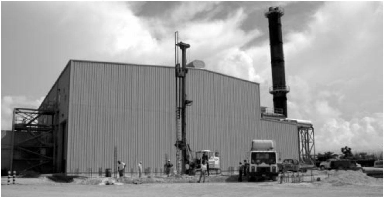
Expansion of Engine Room 5 has commenced to accommodate the new 16 MW V48/60 medium speed diesel generating unit. The unit is scheduled for commissioning in summer 2007.
