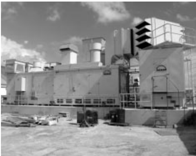
The newly installed 8.4 MW gas turbine is scheduled for commissioning in August 2006.
