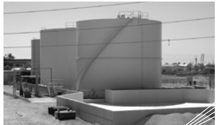
CUC's onsite fuel storage tanks at the North Sound Road Power Plant.
